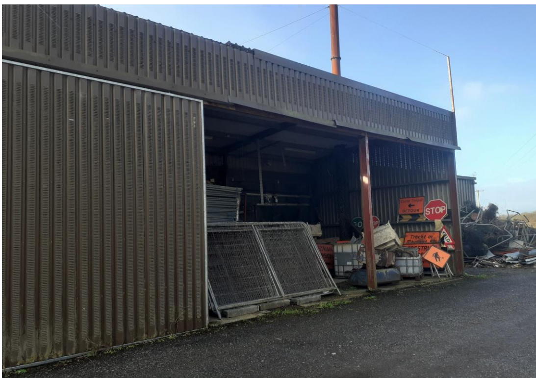
Plate 7. View of commercial units on site – these are metal structures and generally unsuitable for roosting bats (December 2022).
